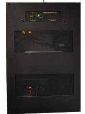
Network Control Hub
