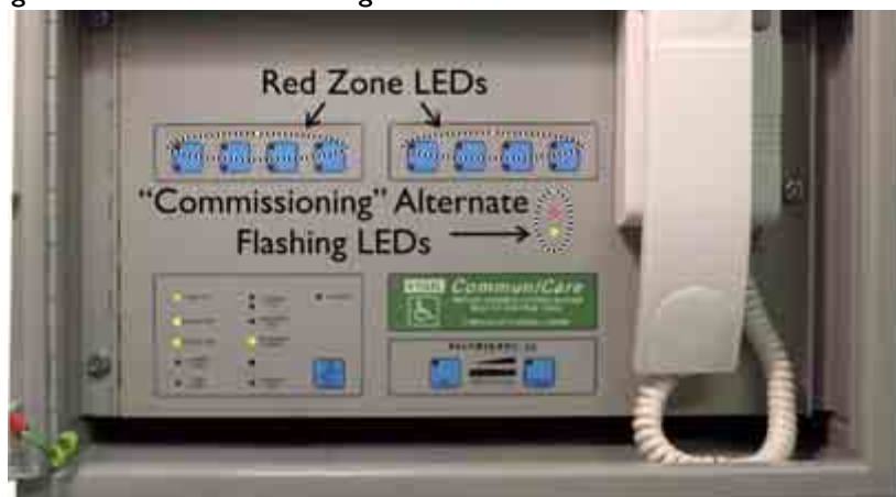
Figure 4.3 — Commissioning Process LEDs
